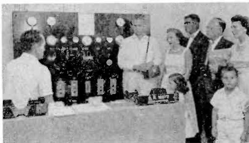
George Mays (left) Building Superintendent giving a run down on the control panel which regulates the heating and air conditioning system throughout our building.
